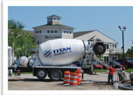
Lewis Witt (pictured right), owner of Inner View, Ltd., very generously donated the installation of our concrete pipes below the park.
